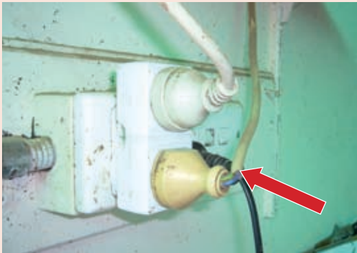
Damaged power leads which have not been inspected and tagged are used.
