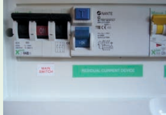
Residual Current Device (safety switches) hard wired into all electrical switch boards.
