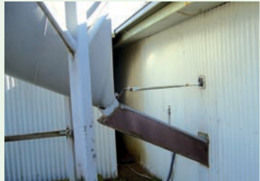
Silo is connected directly to the feed preparation area.
